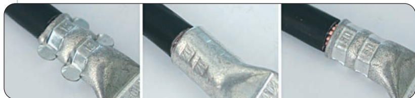
Picture 4: Comparison of incorrect and correct crimps: Faulty crimps (left excess compression, middle low compression) or the use of incorrect crimping tools can lead to increased contact resistance and consequently can endanger the safety of the equipment resp. facility); right = correct crimp
